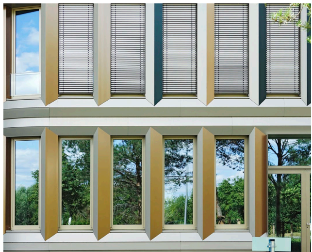
When lowered, external blinds can protect against collisions. However, this is user-dependent and therefore not suitable as a permanent solution.
