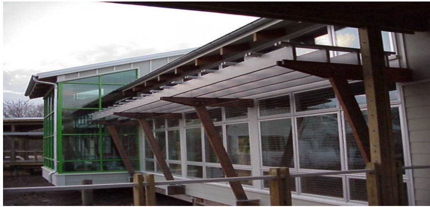
Window netting installed feet from window on slanted wooden beams. Photo by USFWS
